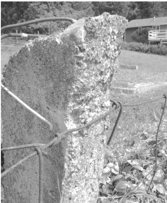
The "back" of a fence post facing south and showing grade 5 (the most severe) weathering near the top. The side facing west (on the left) shows only grade 1.
