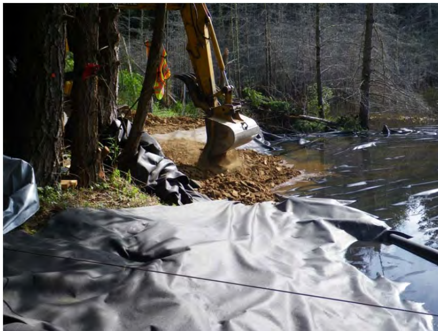
Placement of fill over the geofabric. Note that the geofabric is containing the majority of sediment generated within the immediate construction area.
