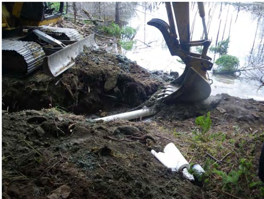
Backfilling trench following breaching of plug at wetland end of the trench and placement of drainage pipe.
