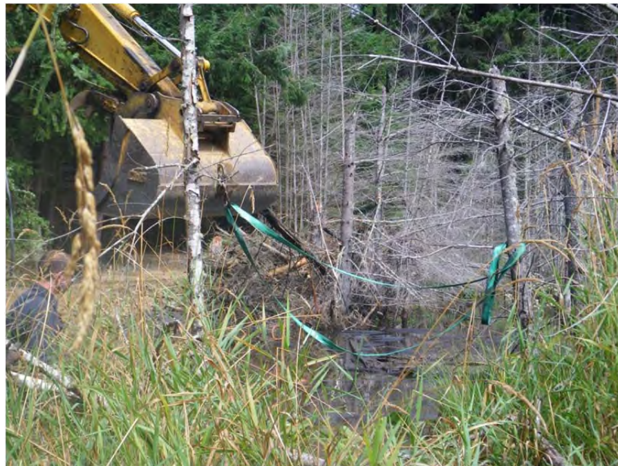
Snags being removed from the berm footprint area with straps attached to the excavator bucket.
