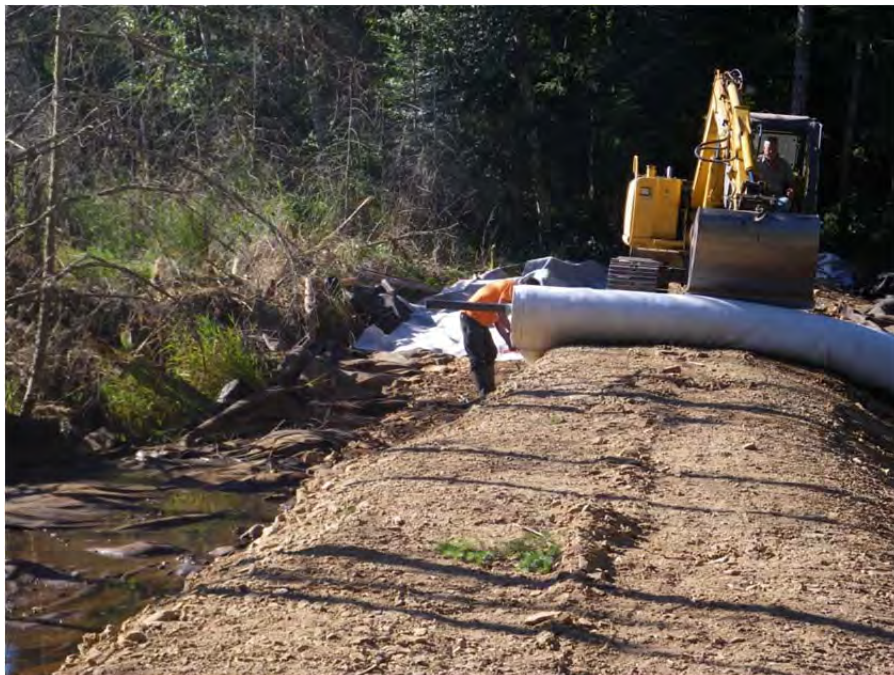
Rolling out geosynthetic clay liner for installation on the wetland side of the berm.
