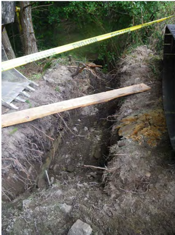
Trench constructed for drainage pipe, connecting to Coats Marsh outflow watercourse downstream of concrete weir.
