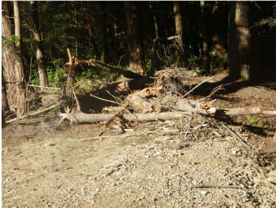
LWD pile placed over the machine turnaround area to the south of the weir.
