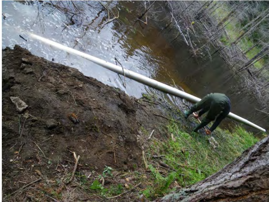
Placing drainage pipe by hand in area to the landward side of the berm.
