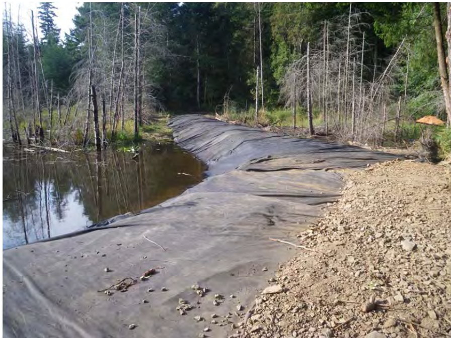
Looking south across the berm following the installation of the clay liner and overlapping with geofabric.
