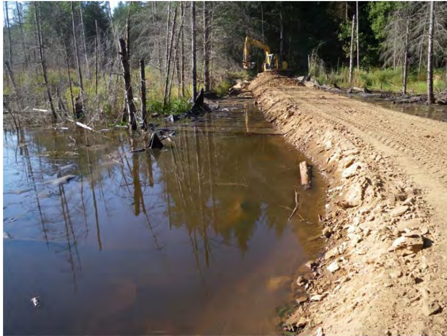
Looking south east across the berm spanning the length of the wetland.
