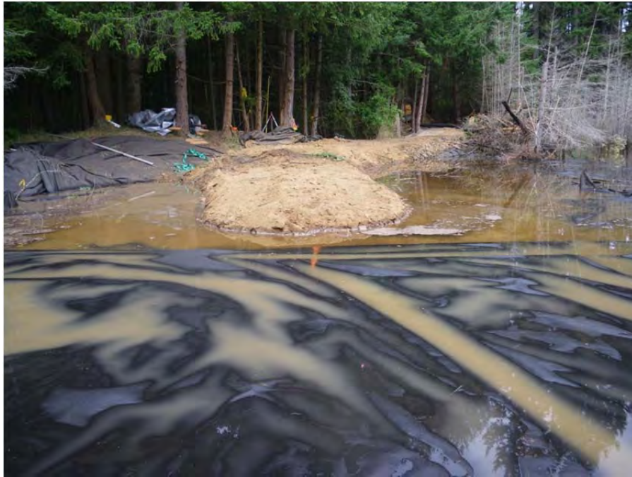
Looking north west along the berm construction footprint area. Note that the geofabric is containing the majority of sediment generated during the fill placement process.
