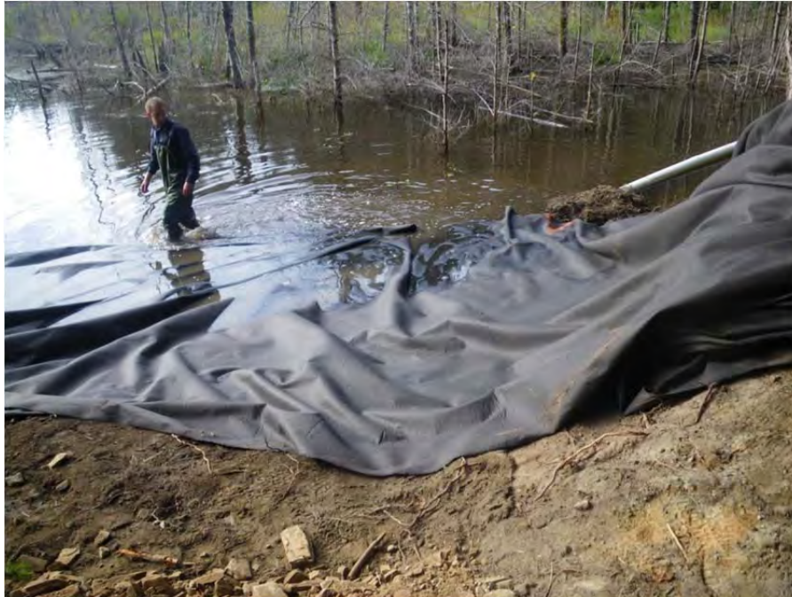
Placing geofabric material over wetted portion of wetland prior to placement of fill.
