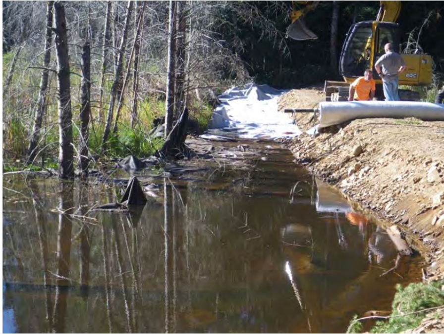
Rolling out geosynthetic clay liner for installation on the wetland side of the berm.
