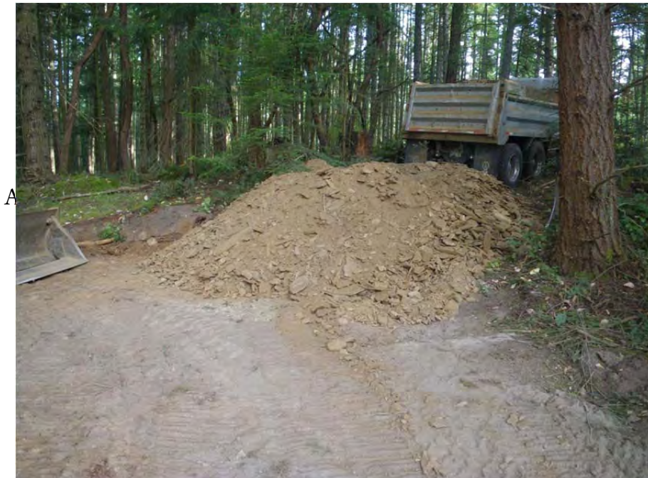
Fill for berm being delivered by dump truck at the end of the access road.
