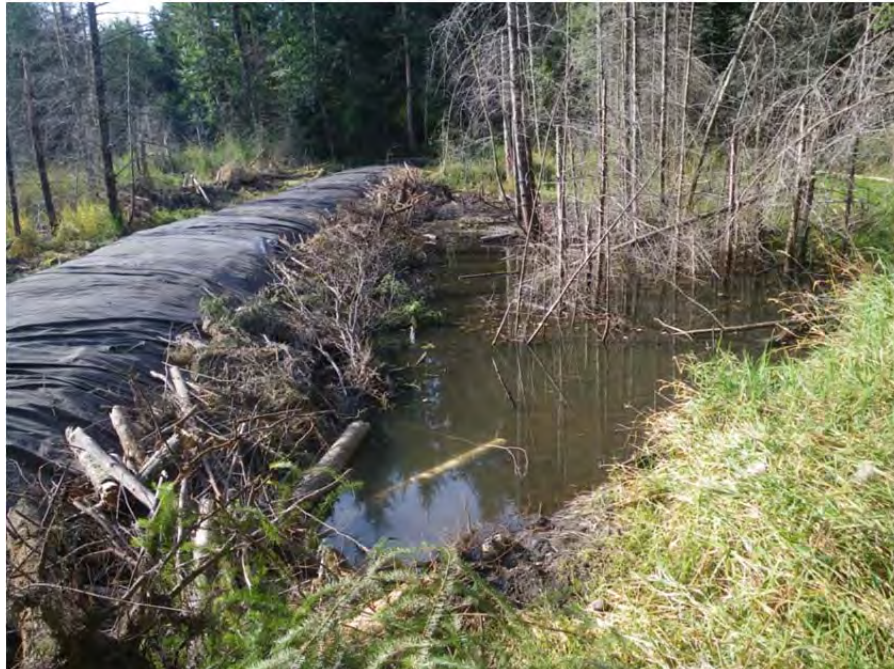
LWD placed along the edge of the berm will provide cover/security habitat for amphibians. Note inlet of PVC drainage pipe in the foreground.
