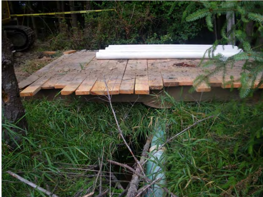
Clear-span steel girder/timber bridge place over outlet drainage and pond leveler pipe to allow machine access.
