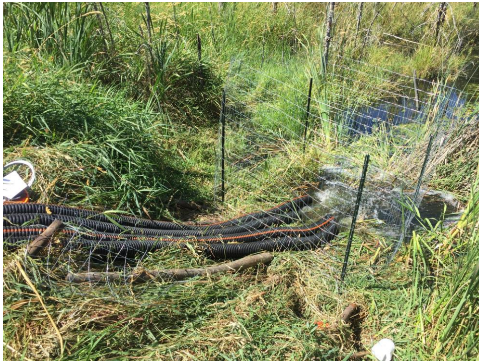
Photo 10. Outlet of temporary draw down siphons. August 4 th , 2021.
