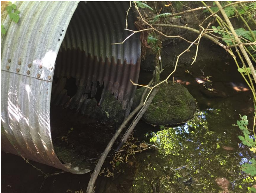
Photo 13. Flow conditions at the inlet of the South Road culvert on Coats Marsh outlet stream on the afternoon of August 4 th , 2021, immediately following influx of flow over the concrete weir and through the leveler. Note lack of turbidity.
