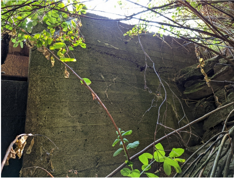
Photo B13 Concrete cracks in weir.
