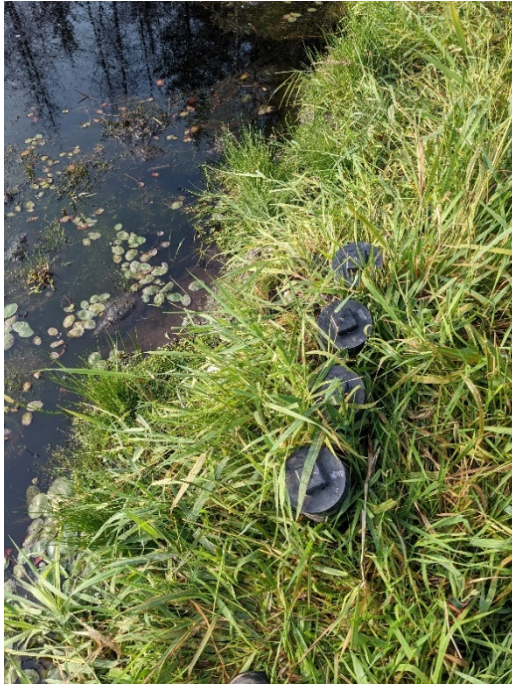
Photo B7 Part of RDN installed siphon system in beaver dam, almost completely obscured by vegetation.
