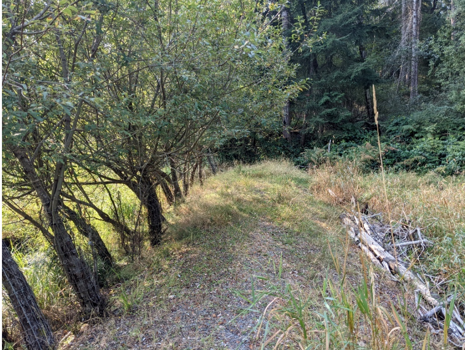
Photo B15 Berm, willows are caged near their bases to prevent beavers from cutting.
