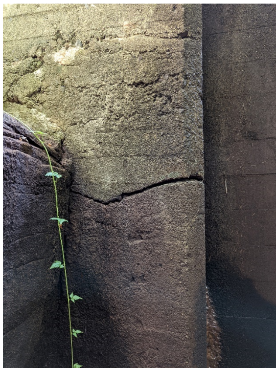
Photo B12 Concrete cracks in weir.
