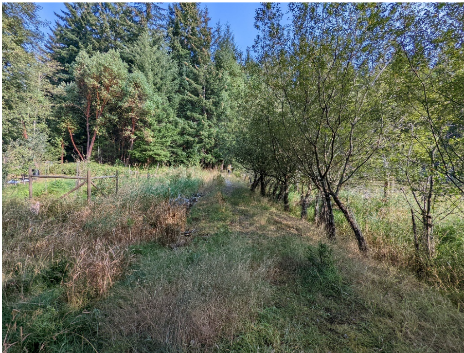
Photo B16 View of berm looking north. Weir pool is on the right and private property to the left. Leakage occurs through the berm, as evidenced by wetland vegetation.
