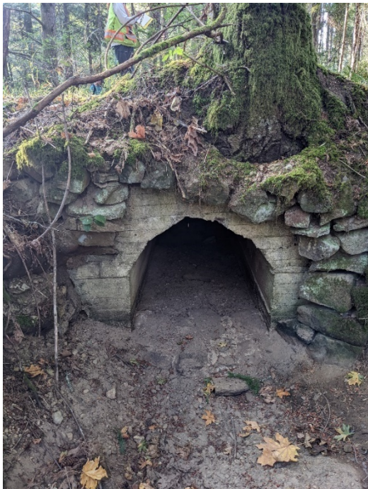
Photo B22 Culvert crossing below easement accessing Coats Marsh Regional Park from the west.
