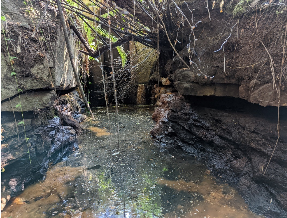
Photo B19 View in the narrow channel immediately downstream of the weir.
