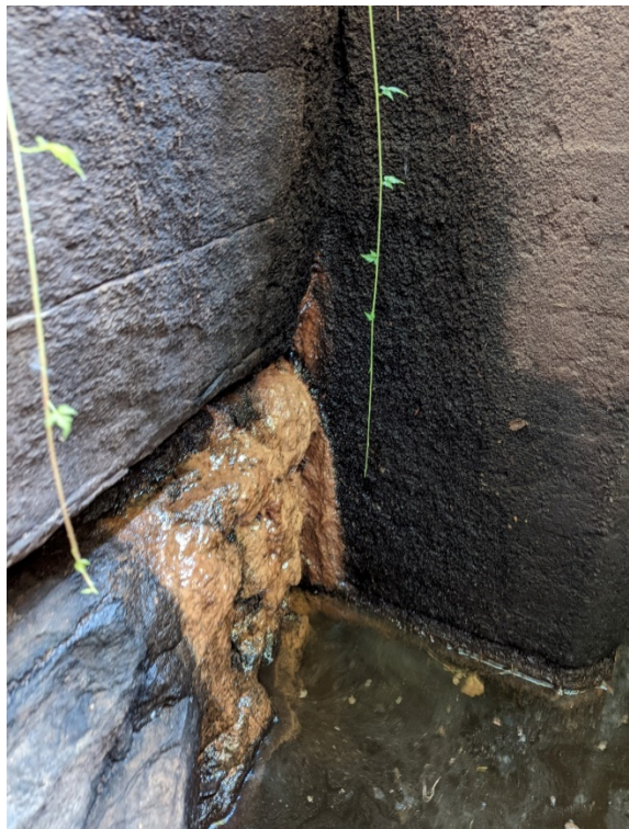
Photo B11 Leaks visible in the weir structure from downstream.
