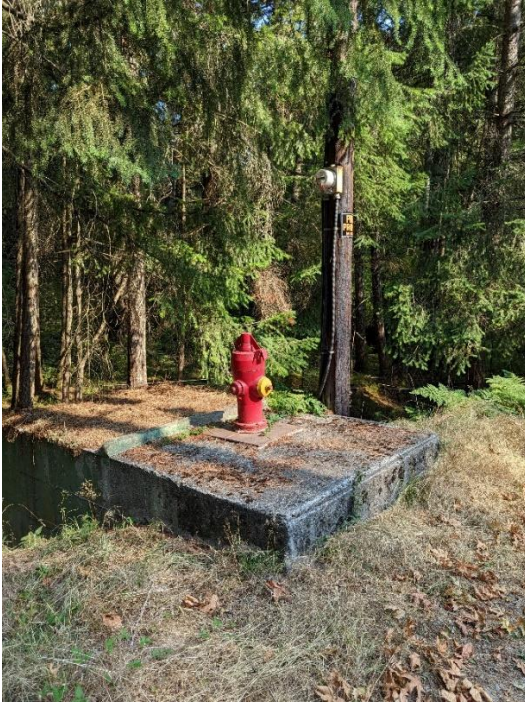
Photo B25 Fire hydrant and pump house located at South Road near Coats Marsh Creek (14 Sept 2022).
