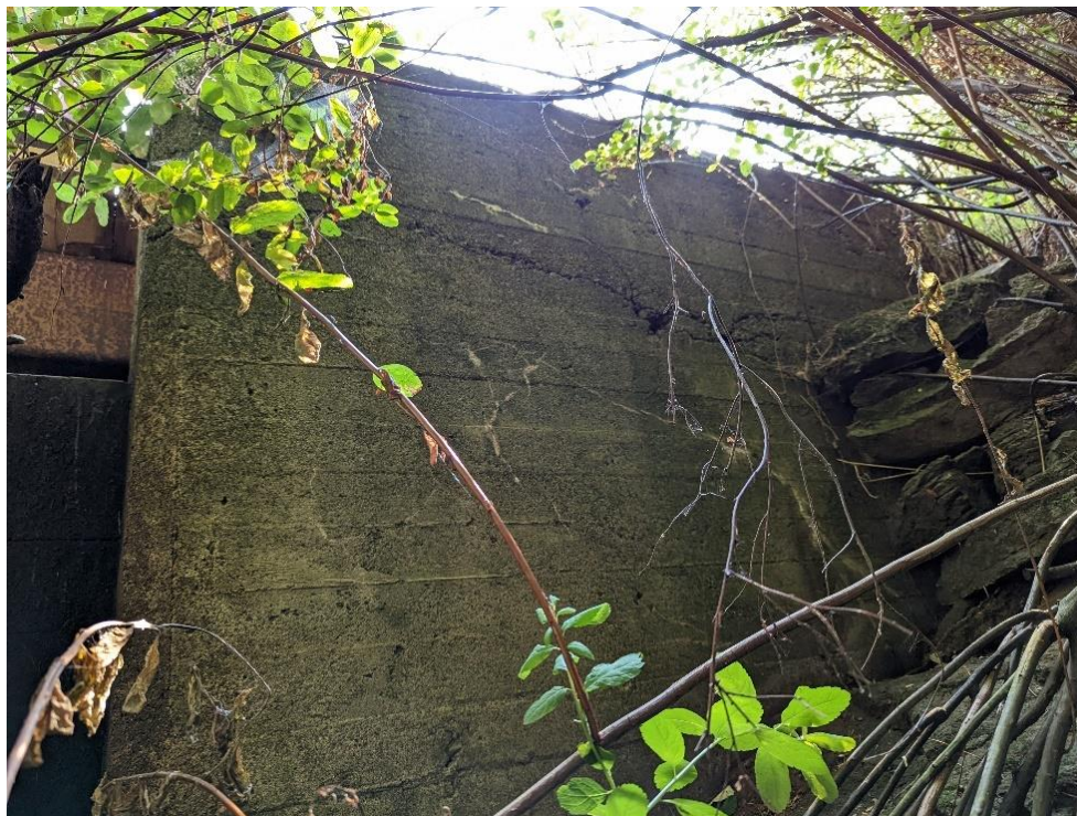
Photo B13 Concrete cracks in weir (14 Sept 2023).
