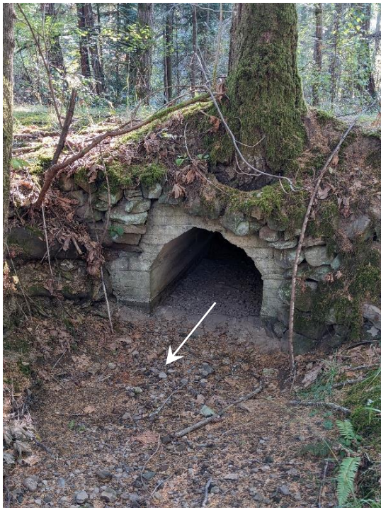
Photo B22 Culvert crossing below easement accessing Coats Marsh Regional Park from the west (22 Sept 2023).
