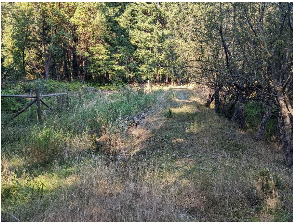
Photo B16 View of berm looking north. Weir pool is on the right and private property to the left. Leakage occurs through the berm, as evidenced by wetland vegetation (22 Sept 2023).
