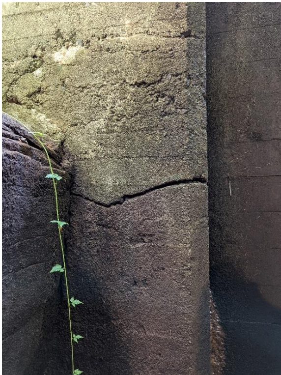
Photo B12 Concrete cracks in weir (14 Sept 2023).
