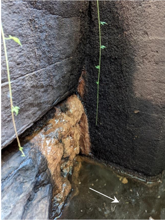
Photo B11 Leaks visible in the weir structure from downstream (14 Sept 2023).
