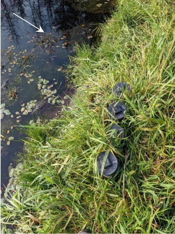
Photo B7 Part of RDN installed siphon system in beaver dam, partially obscured by vegetation.
