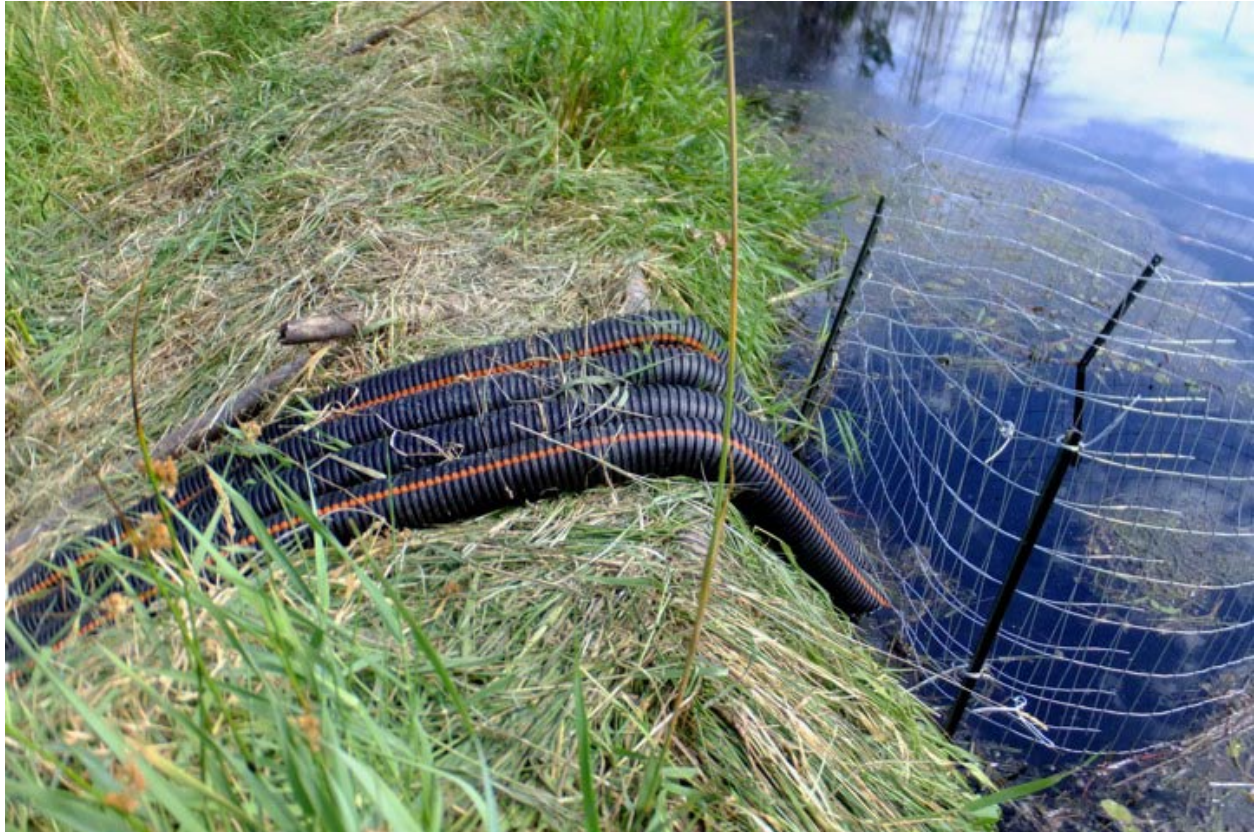
Syphon intake: [4 hoses 5"OD, 0.8m head, ~87 L/s total; my guess, simulating a 200mm ID PVC pipe]
