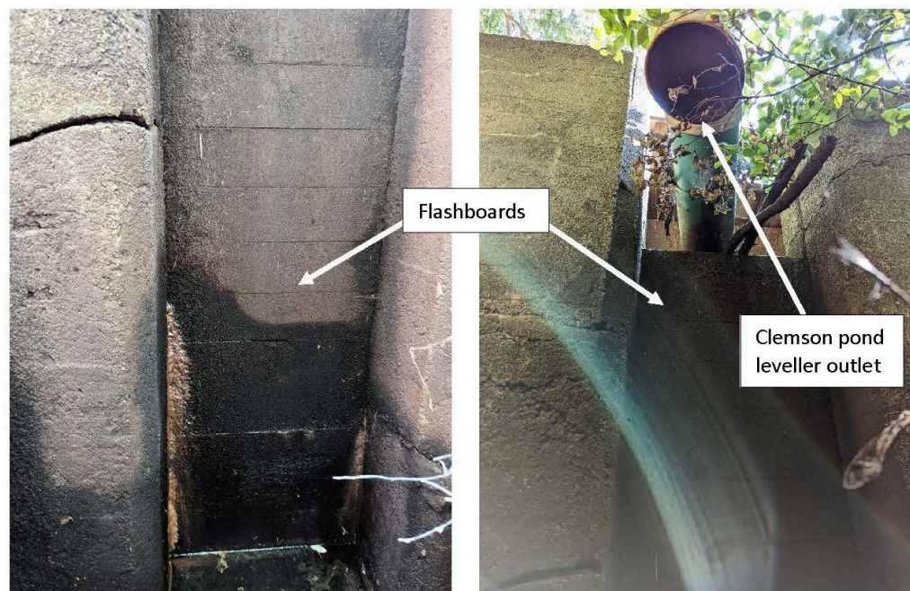
Photo 2.4 Lower (left) and upper (right) portions of the weir outlet slot and flashboards, viewed from the downstream channel. Note cracks in the concrete at several locations (NHC, Sep. 2022).
