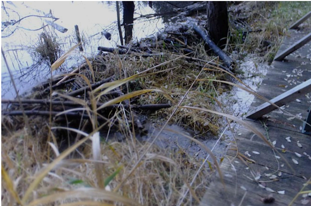
The debris/dam at the weir, December 8, 2023. More than one engineer been working on it ?
