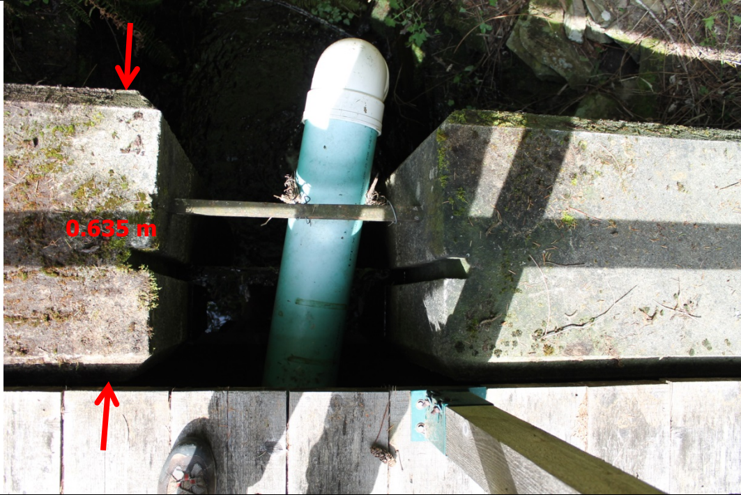
27. View looking down on weir crest and stop-log controlled spillway; 200mm pond leveler pipe visible
