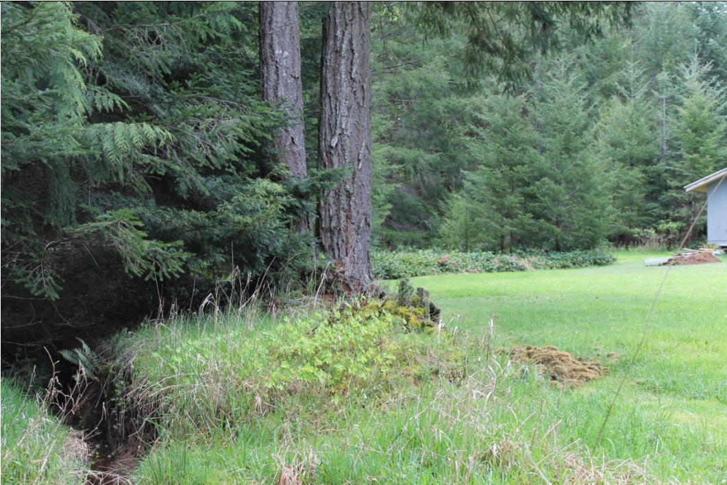
76. View showing spill channel at left and grassy left bank – terrain gently slopes up to right
