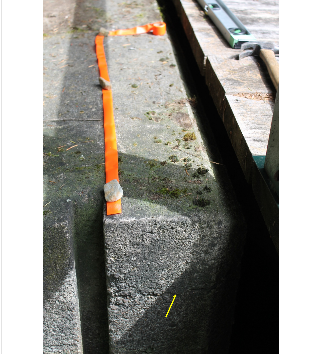
23. Opposite view of area of spalled concrete on right crest of weir – note deep spall crack (yellow arrow)
