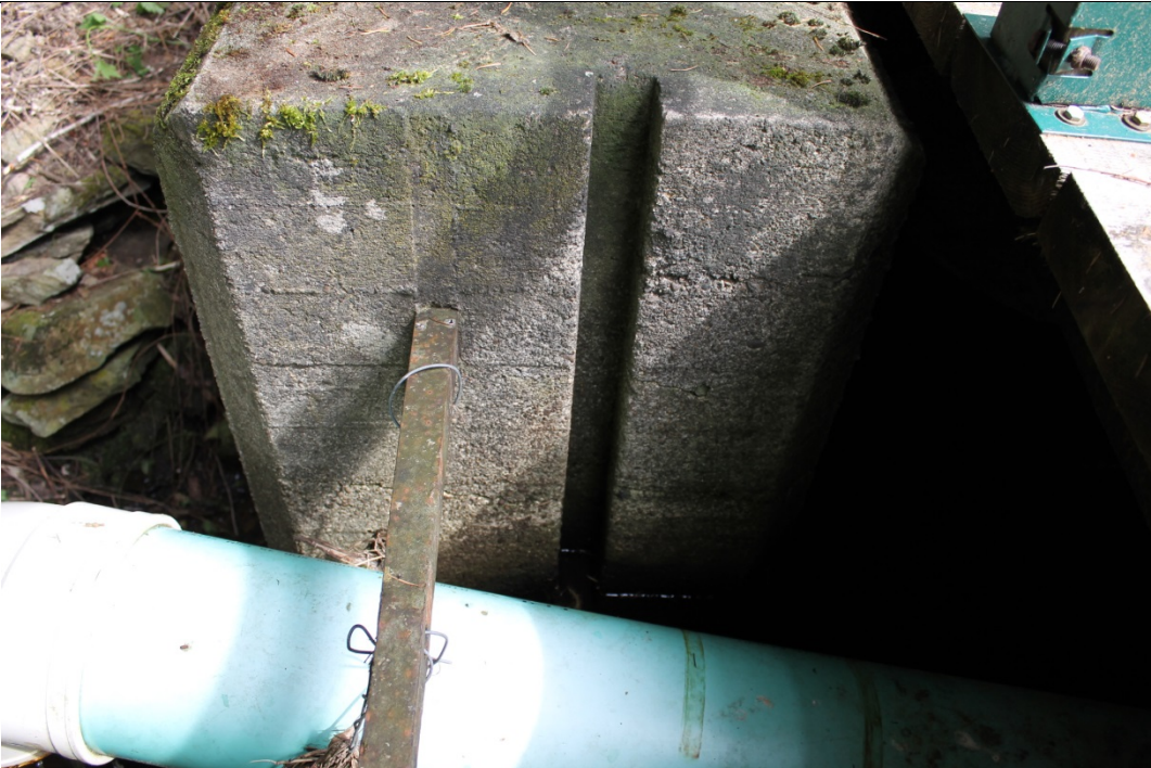
38. View of spillway, looking toward right abutment – stop-log gap in concrete and 200mm pond leveler pipe visible
