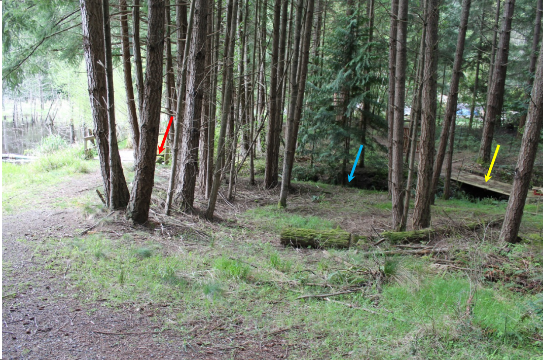
40. Concrete weir (red arrow), blasted spillway channel (blue arrow) and residential property owner bridge 1 (yellow arrow)
