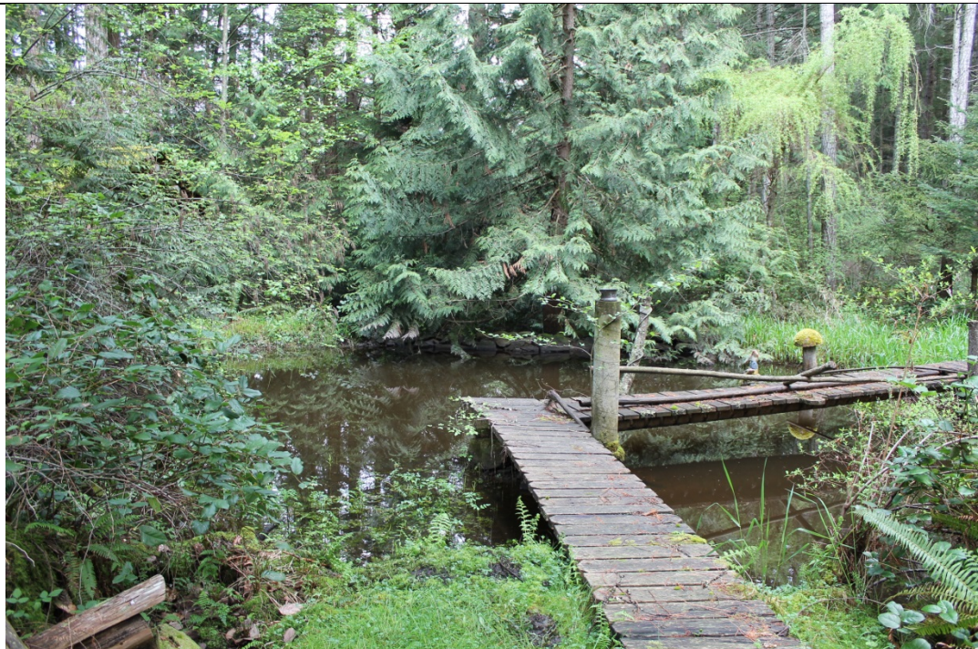
52. View of foot bridge 2 looking from left bank to right bank of spill channel – very flat terrain
