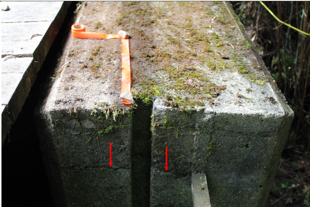
26. Opposite view of area of spalled concrete on right crest of weir – note deep spall crack (red arrows)
