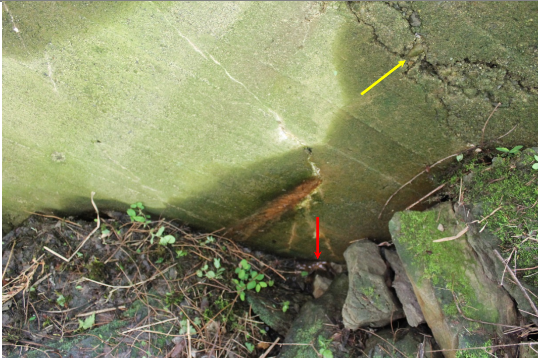
36. D/S face of concrete weir at left abutment & close-up of potential dry joint/honeycomb (yellow arrow) & minimal seepage (red arrow)
