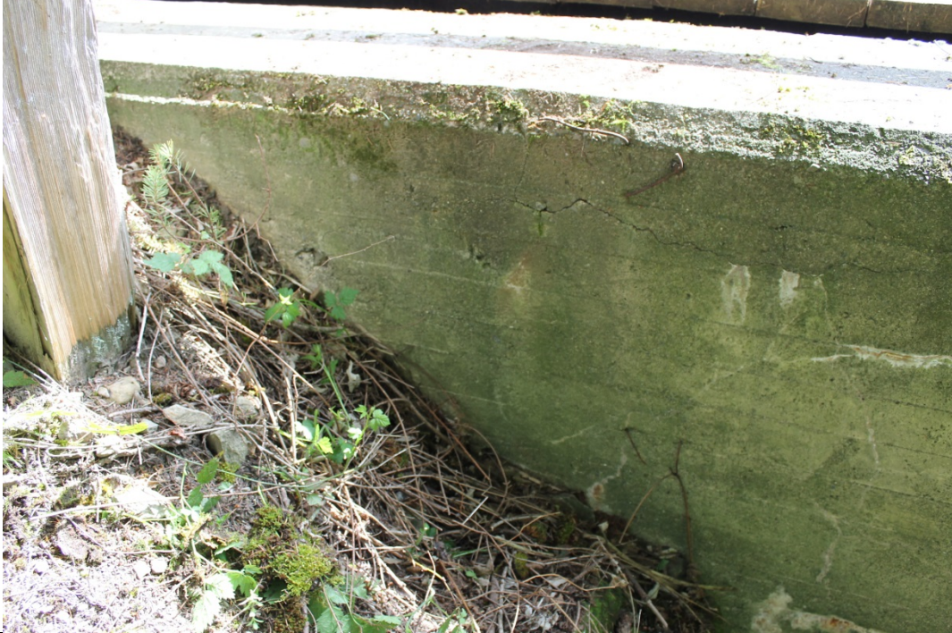
31. D/S face of concrete weir near right abutment – many cracks visible
