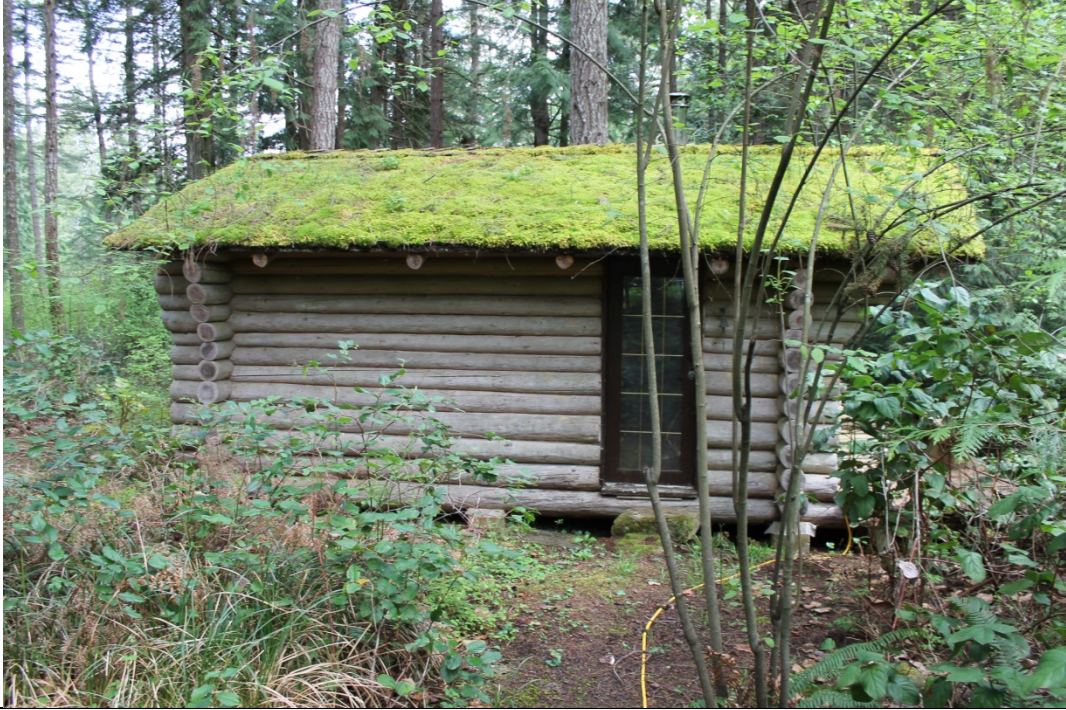
55. Side view of uninhabited recreational cabin – part of property at 1040 Coats Drive
