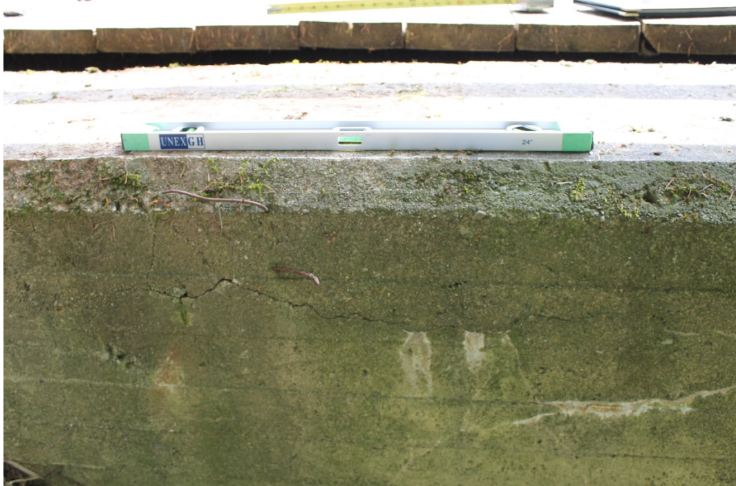
32. Close-up of photo 21 showing length of most obvious crack near top of concrete weir (24" long spirit level on crest)
