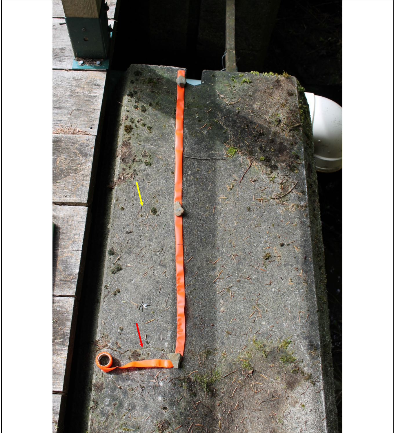
22. Area of spalled concrete at right crest of weir (taped area below yellow arrow) – note top crack (red arrow)
