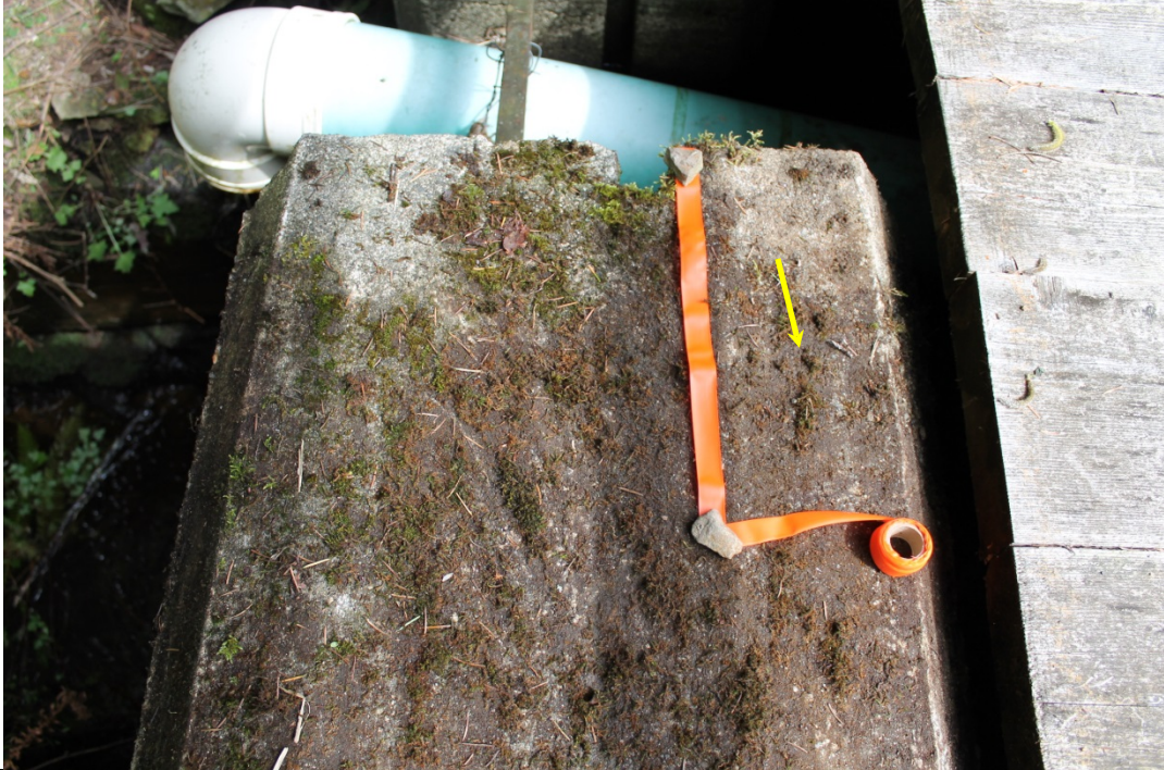
25. Area of spalled concrete at left crest of weir (taped area below yellow arrow)
