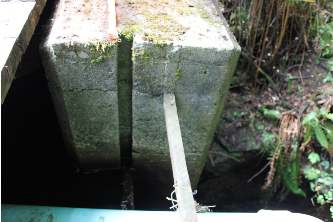
37. View of spillway in center of concrete weir, looking toward left abutment – stop-log gap in concrete
