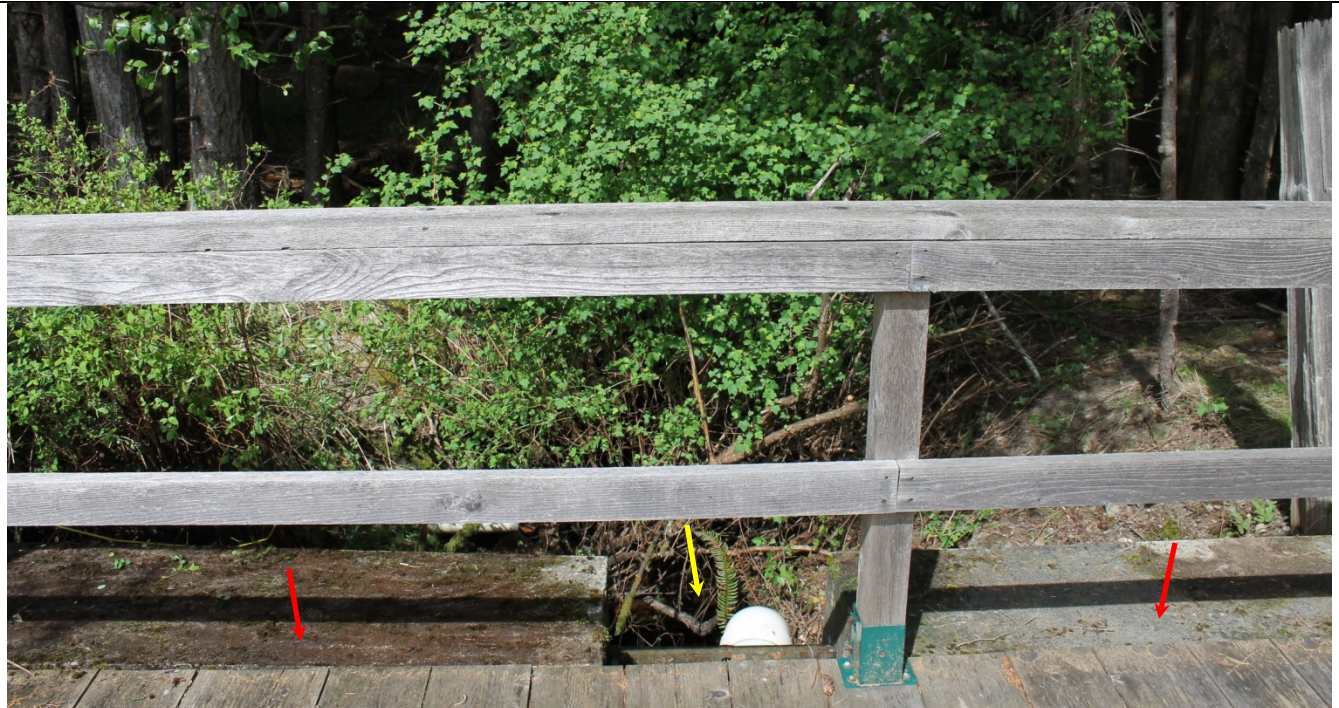
14. U/S view of concrete weir (red arrows) looking downstream past spillway gap (yellow arrow)
