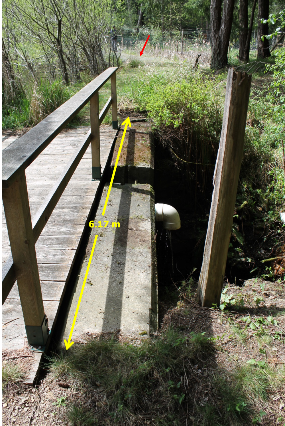
19. Concrete weir crest viewed from right abutment; residential property protection dyke in background (red arrow)
