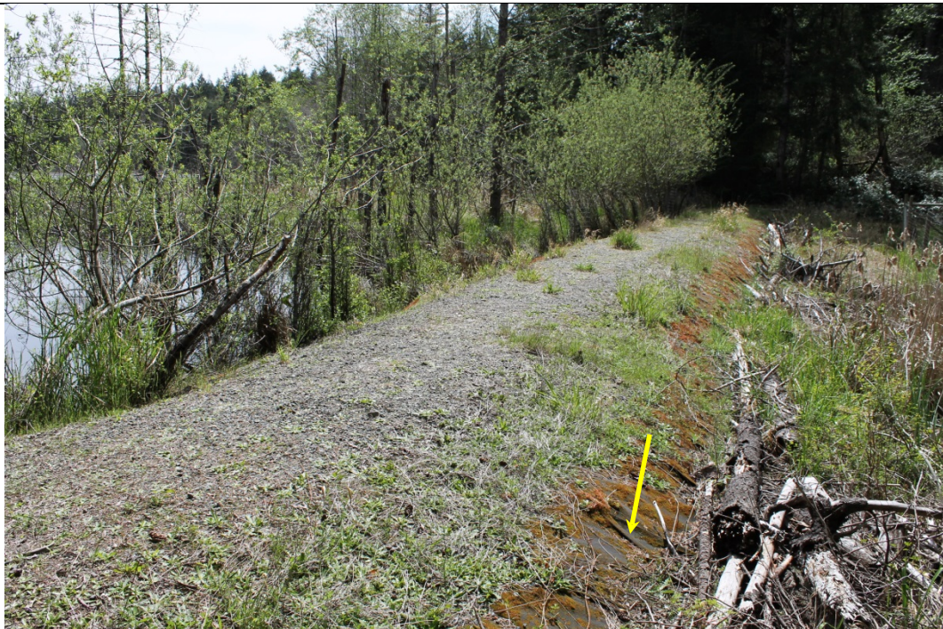
6. Residential property protection dyke – willows planted on U/S side, visible geotextile covers entire berm (yellow arrow)
