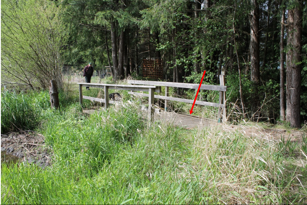
13. U/S view of concrete weir (at red arrow), showing right abutment area
