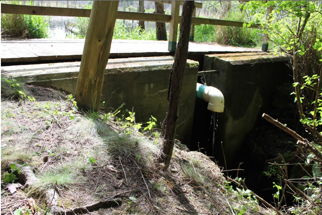
28. D/S view of concrete weir from right abutment – weir is located in a channel blasted into the sandstone bedrock
