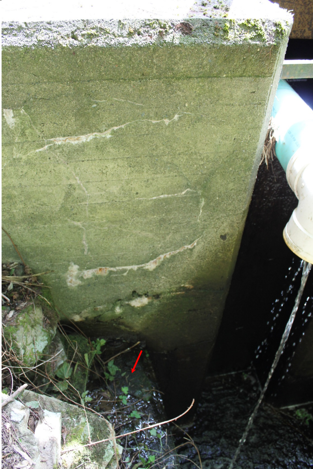
33. D/S right face of concrete weir beside spillway/stop-logs – many cracks and obvious seepage (red arrow) visible
