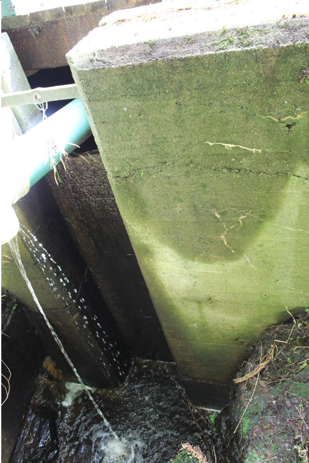
39. View of 41.3 mm thick X 723.9 mm long stop-logs. Stop-logs appear to be sound based on screwdriver probing
