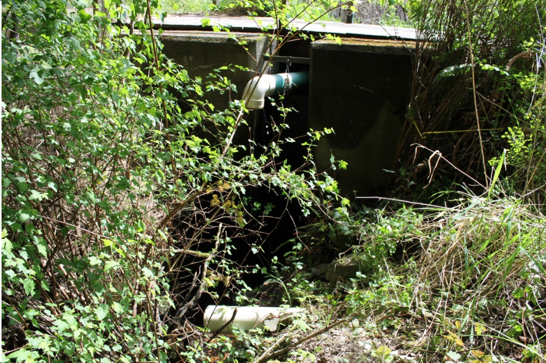
29. D/S view of concrete weir from left abutment; white dyke downstream drain pipe in foreground (see photos 5/6/17 for dyke view)
